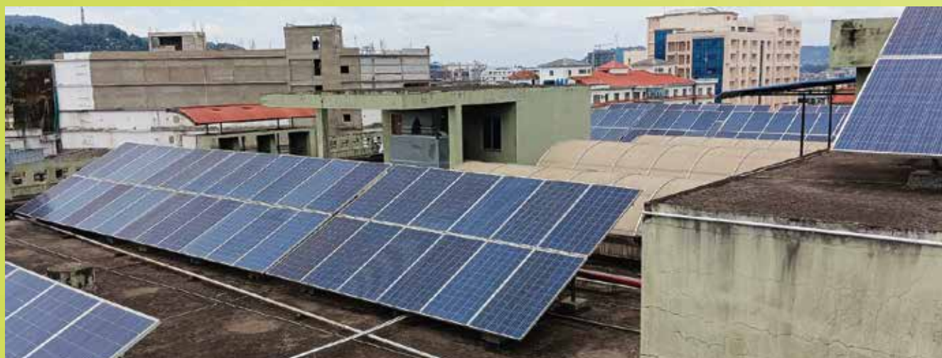
70 KW Solar Plant installed in the Head Office premises
